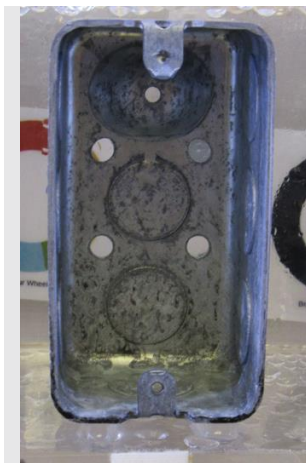
Figure 23. Junction Box, Day 14, Fresh Water.
